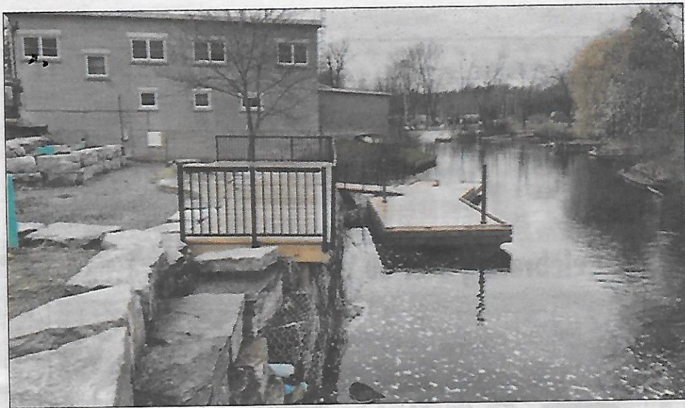
New docks were installed on Mill Creek as the Township of Rideau Lakes continues with development of the waterfront park.
